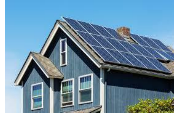
Solar Panels attached to a residential roof
