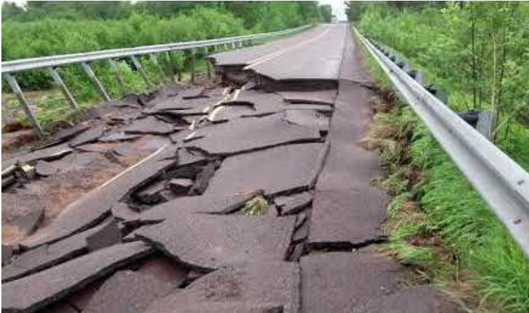
Road conditions in Houghton after the storm.
